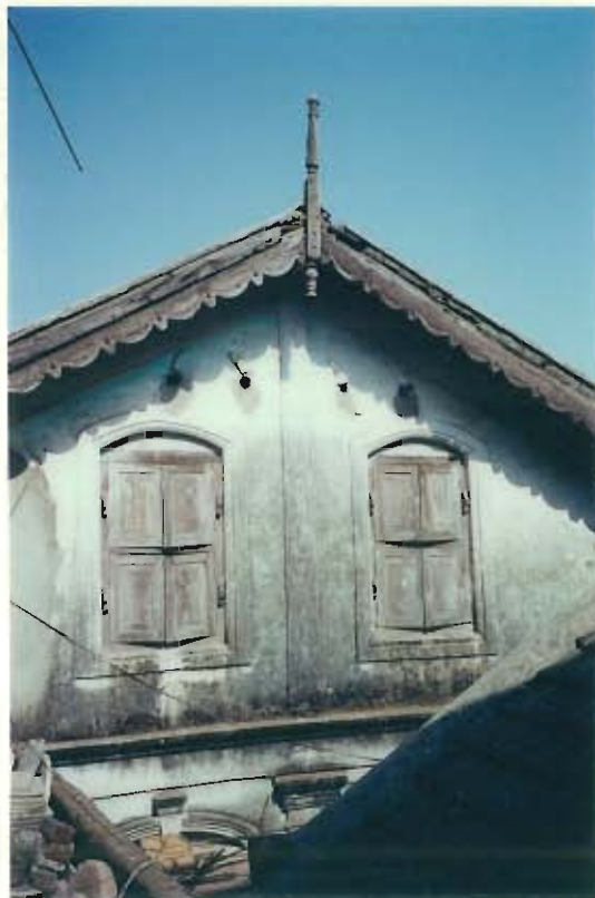
View of the windows of attic space and the gable end of Bhawan Bhavan as viewed from neighboring structure
