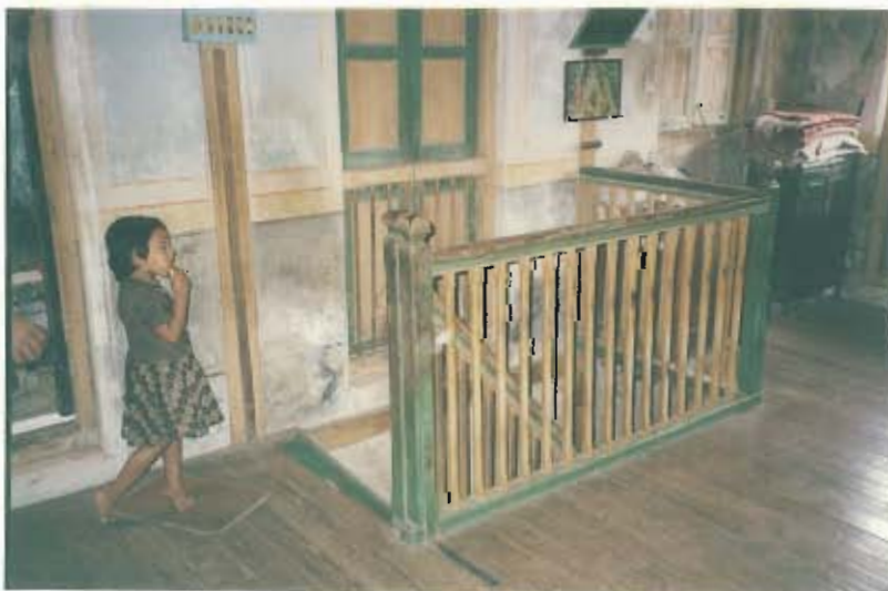
View of the internal staircase with Structural frame and flooring in timber
