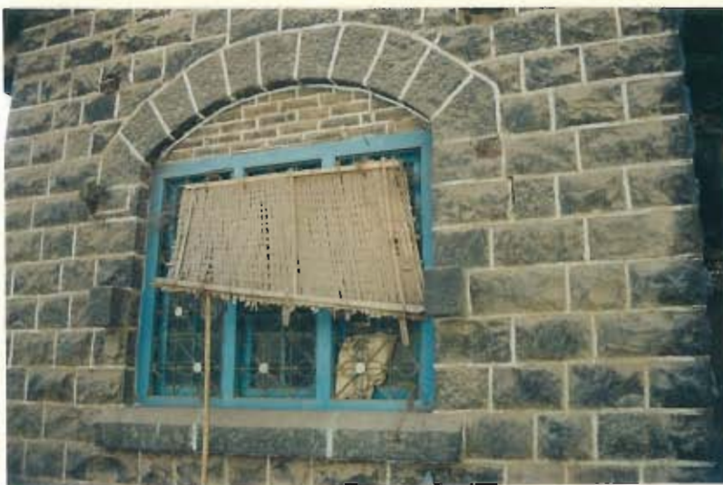
Typical window with stone masonry wall, arch and space infill with brick
