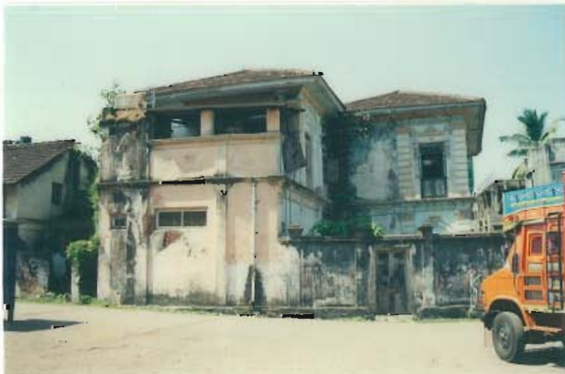
Side view of the structure from Zakir Hussain Chowk - a north east view.
