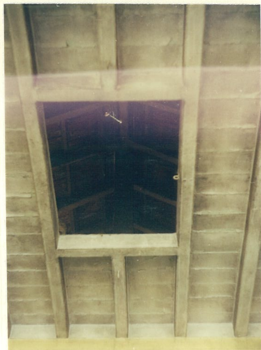
Details showing timber boarding laid on timber joists with an opening to reach attic space with mobile ladder.
