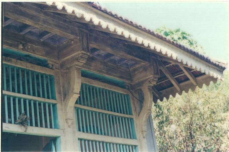
View of ornated timber brackets supporting hipped roof beams and decorative eaves boards in timber with projected Mangalore roof tiles
