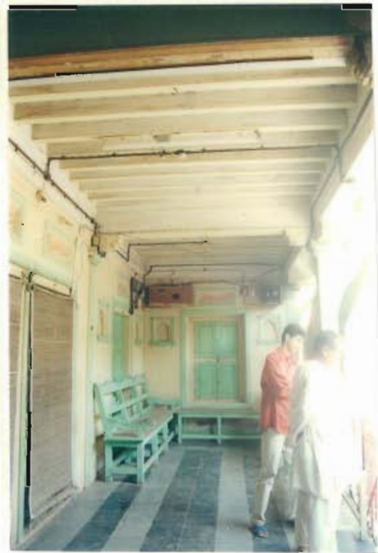
View of the timber joists supporting upper floor boarding and also shows articulated window corners
