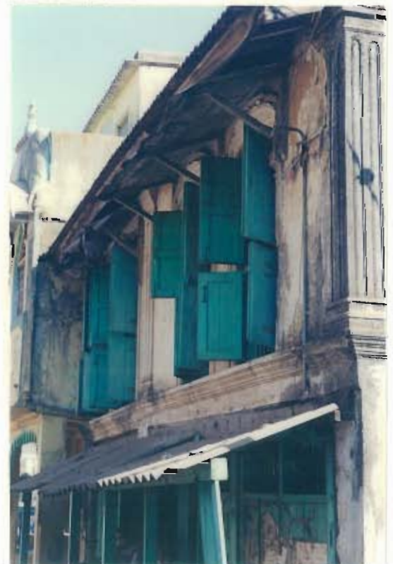
View of a Kanya Shala building from Wani Aali and open space junction.
