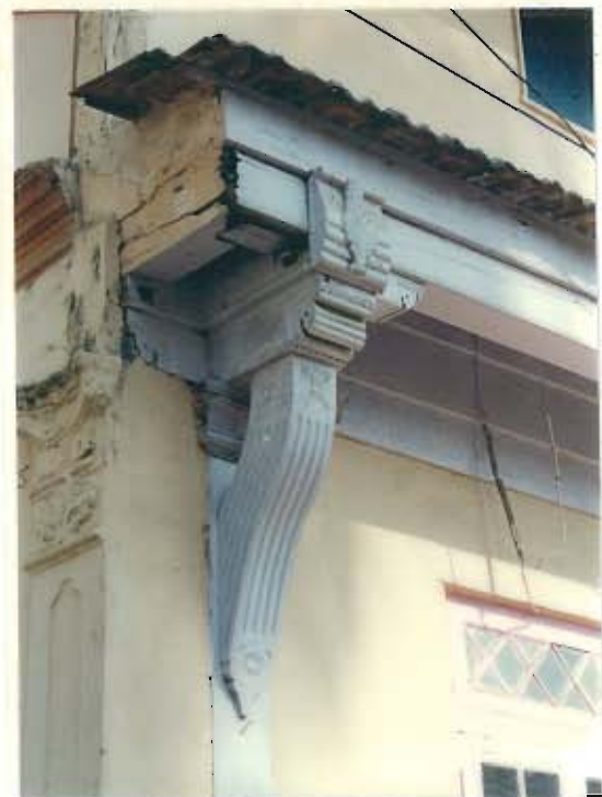
View of the timber bracket with decorative carvings supporting the floor projection above
